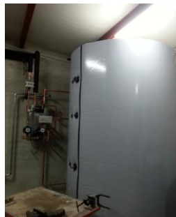
Boiler a biomasse
